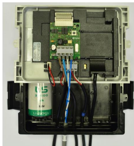
Picture 5.6 - Example of correctly wired module
